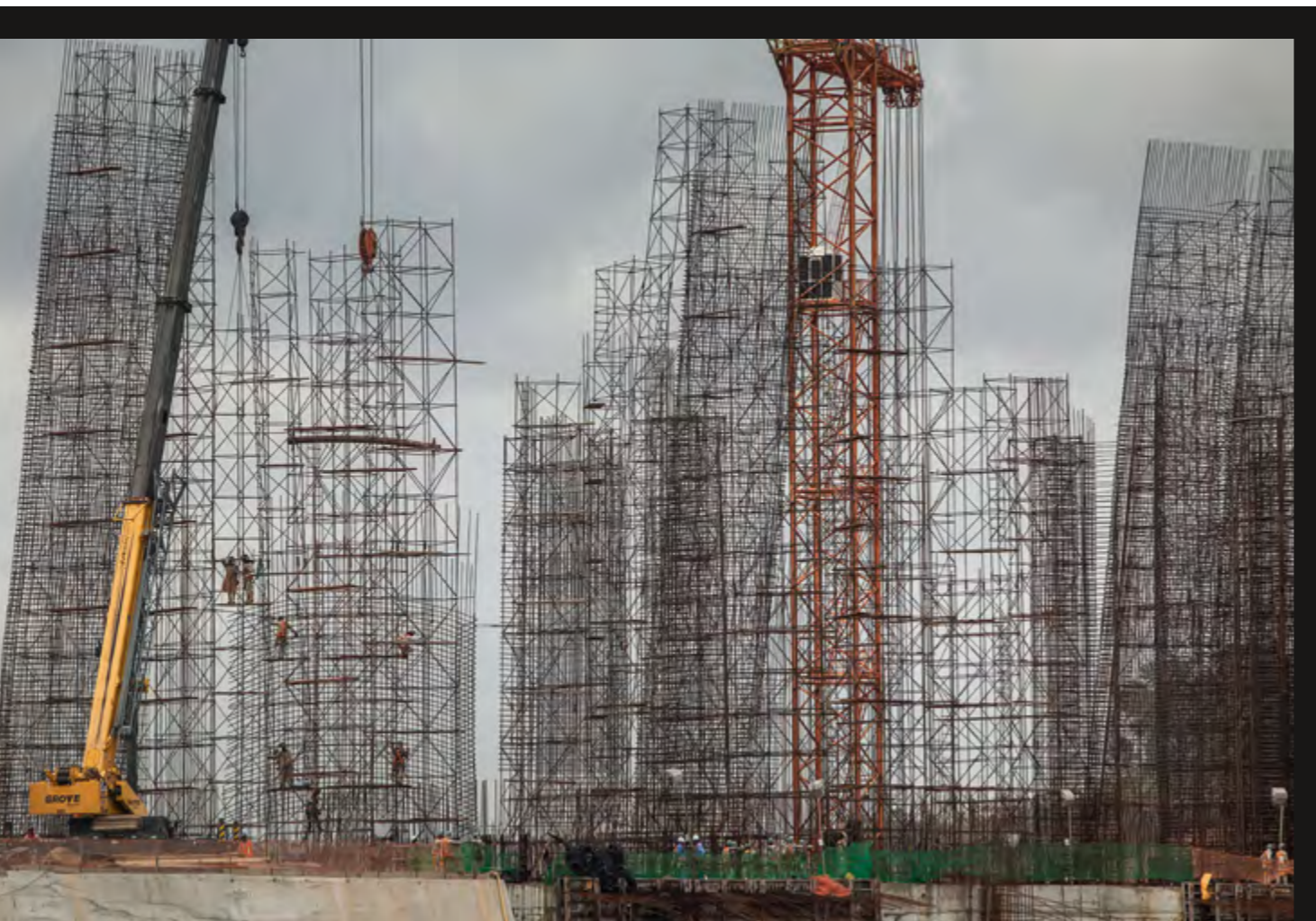
Construction site of the Belo Monte hydropower dam complex, Pará State. © Carol Quintanilha/Greenpeace
