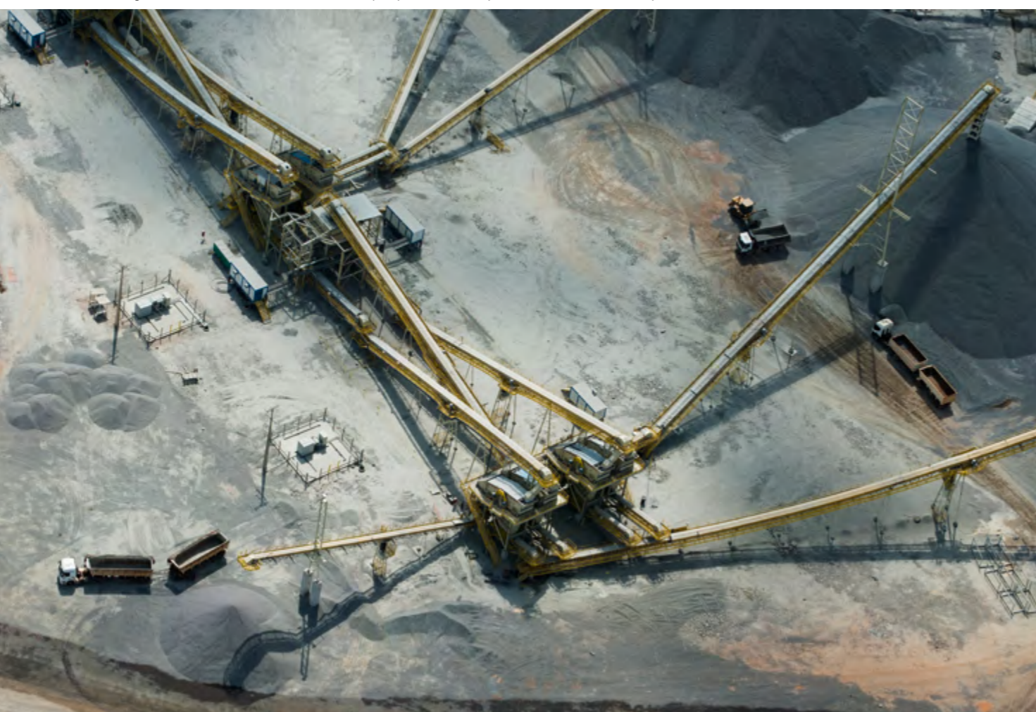
Below / Right: Construction site of the Belo Monte hydropower dam complex. © Daniel Beltrá/Greenpeace
