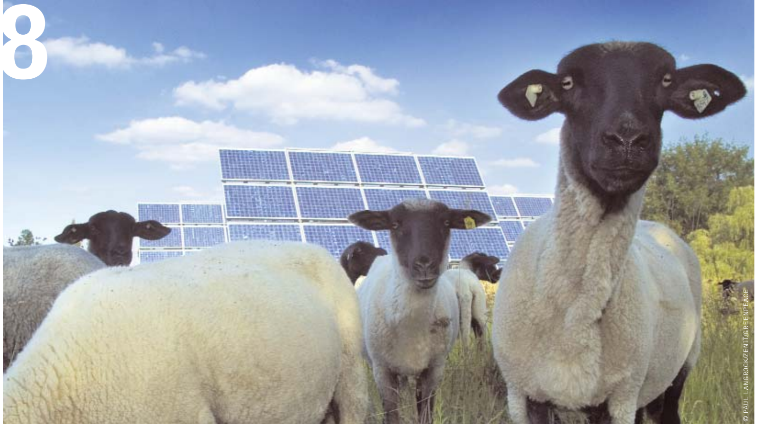
image image PHOTOVOLTAICS FACILITY AT 'WISSENSCHAFTS UND TECHNOLOGIEZENTRUM ADLERSHOF' NEAR BERLIN, GERMANY. SHEEP BETWEEN THE 'MOVERS' KEEPING THE GRASS SHORT.
