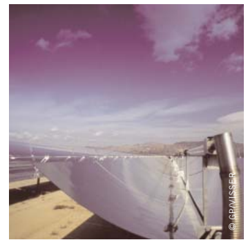
image CONCENTRATING SOLAR POWER (CSP) AT A SOLAR FARM IN DAGGETT, CALIFORNIA, USA.
